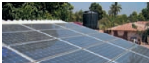
PV generator in Gambia
